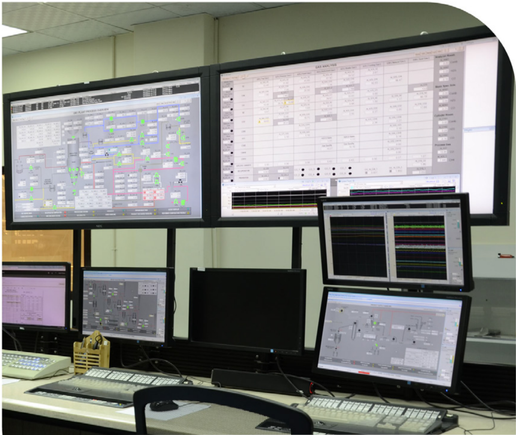
DR Control Room
